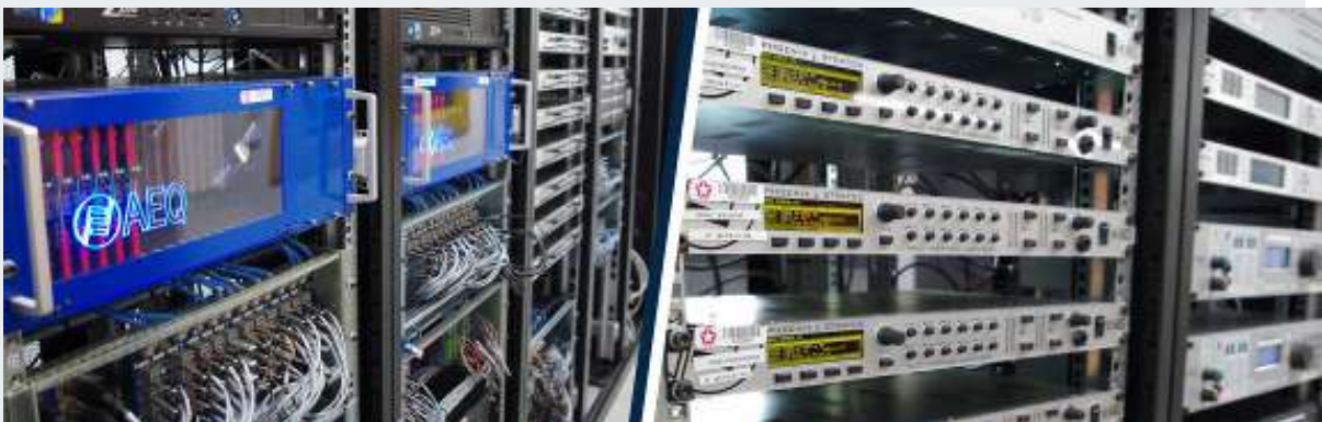
Central Control Room equipment: ARENA audio engine, computers and audiocodex
